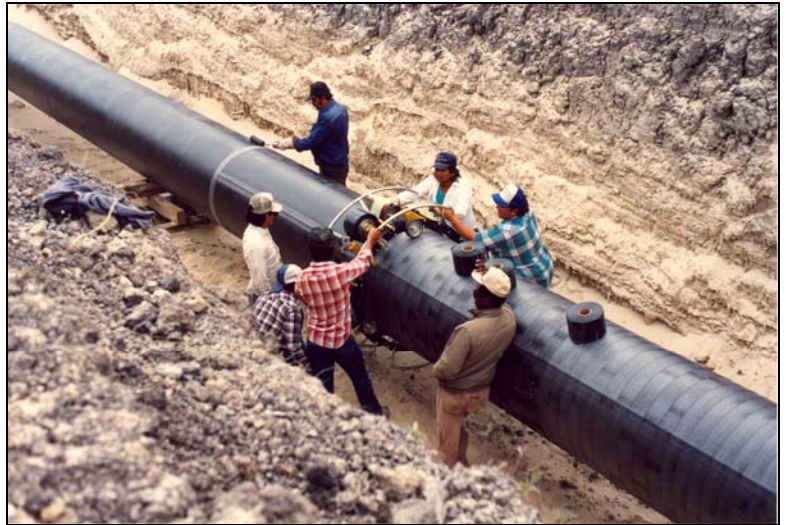
Application of RD-6 by machine is strongly recommended wherever possible. The increased tension of machine application assists in resisting soil stress.
