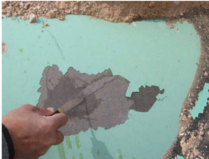
This disbonded FBE had no corrosion underneath. The pH of the water under the blister was elevated (made more alkaline) as the result of the CP currents being able to reach underneath the disbondment.
